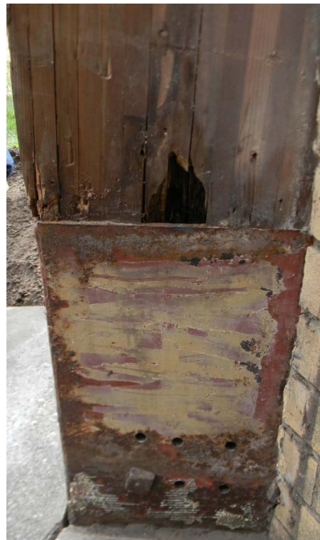
Figure 2 - Timber arch rot inside support shoe
