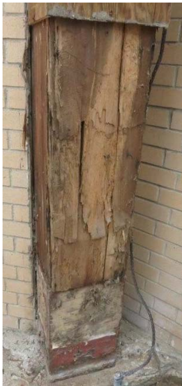
Figure 1 - Timber arch delamination
